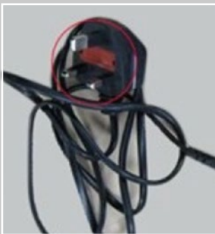
△ Example of incorrect plug pins.
